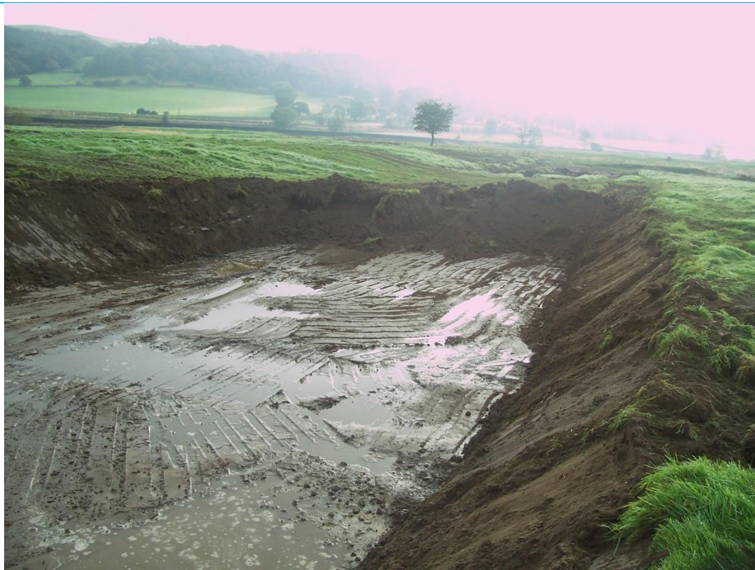
a) Upstream chute channel during construction looking downstream showing fine sediment on bed.
