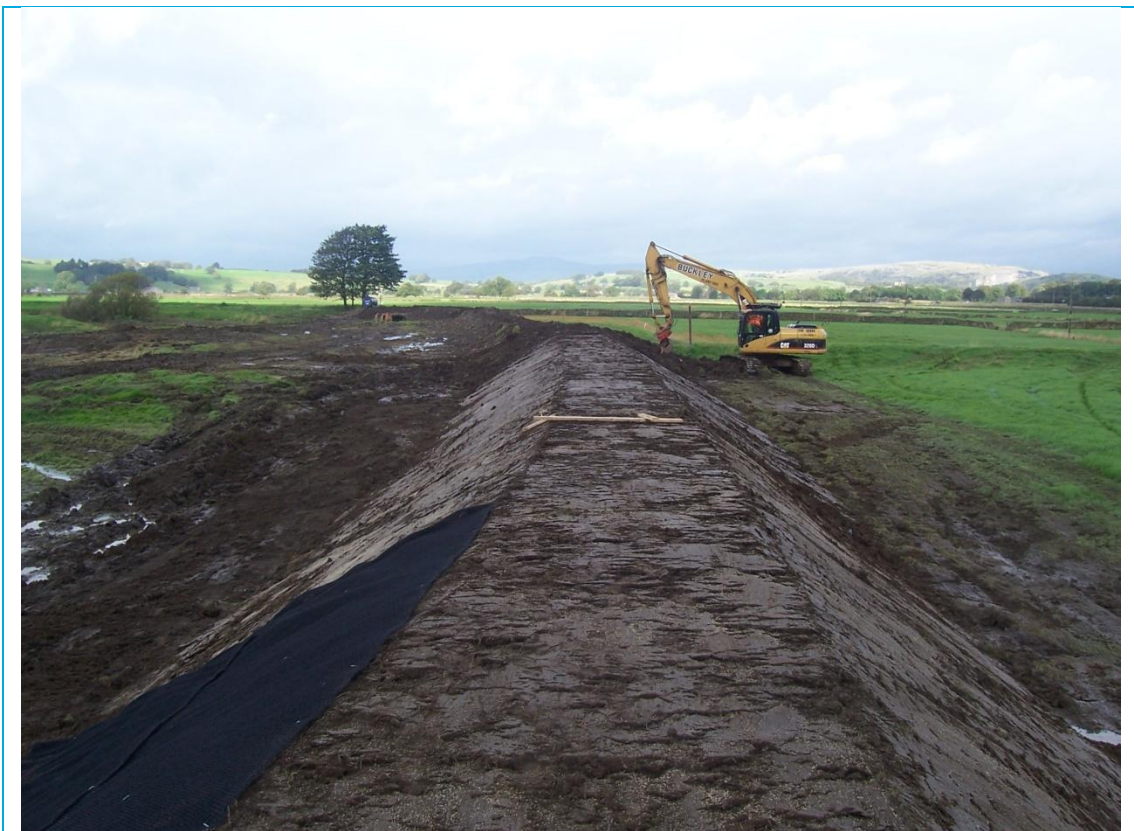
a) Set back flood embankment during construction, looking upstream. Note the flood embankment has been set at a slightly higher level to the original embankment to allow for settlement.
