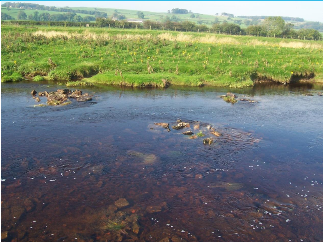
a) Some of installed boulder clusters and general coarsening of the bed towards the left bank
