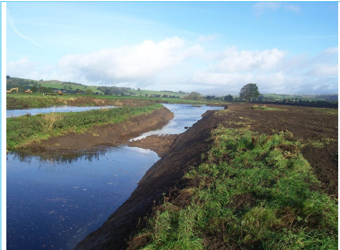
c) Chute channel activated at higher flow, looking upstream. Some sediment deposition was evident after this event.
