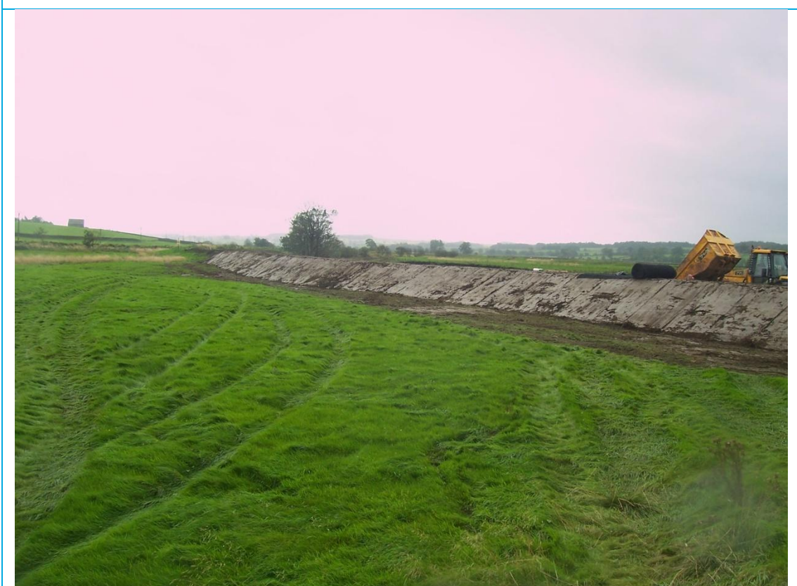
b) View of flood embankment from floodplain side. Seeding was undertaken during the
